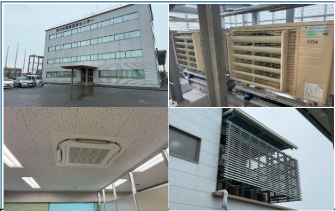
Energy Conservation in the Administration Building(Air-Conditioning System)
