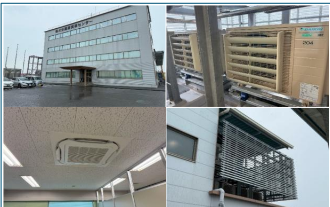
Energy Conservation in the Administration Building(Air-Conditioning System)
